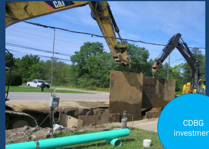
Sanitary sewer line Canton Township
